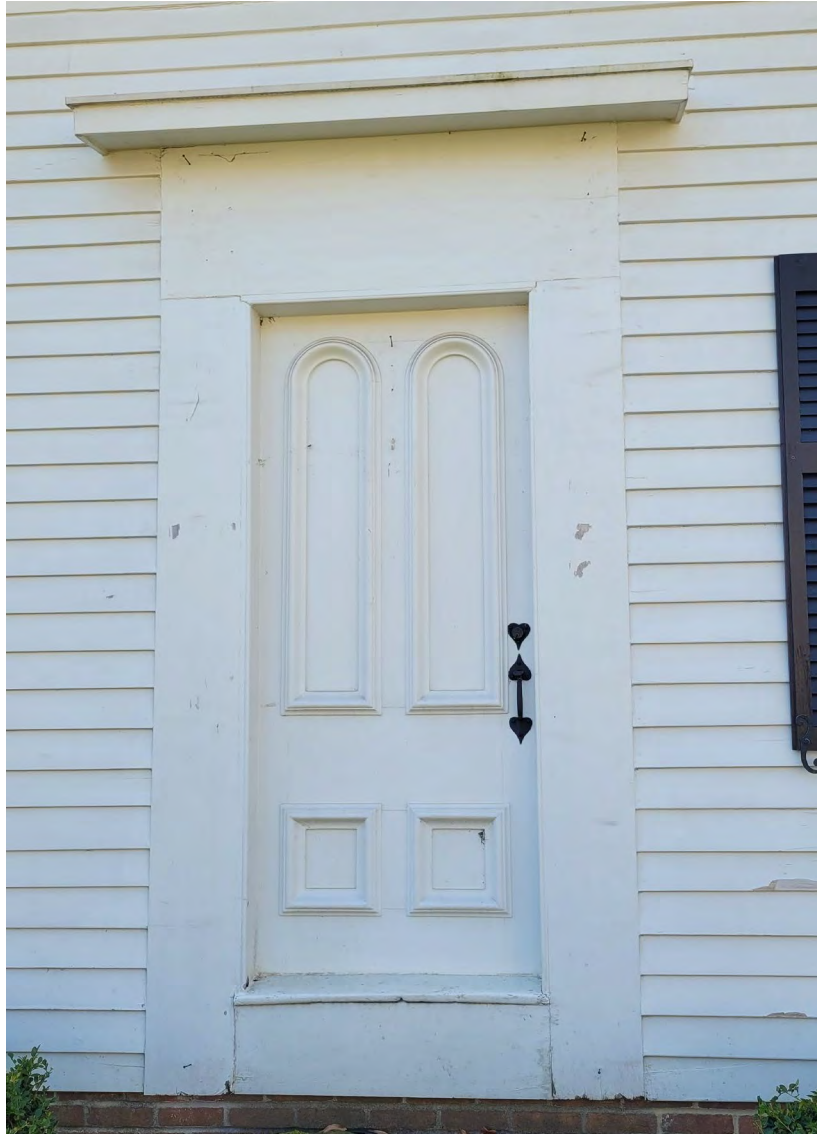
Image 15: Front door, which appears to be a non-historic flush door with applied decoration.
