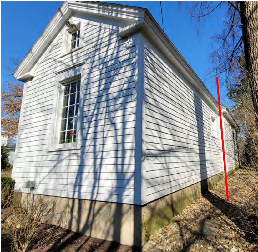
Image 8: Rear (south) and side (east) elevations of the garage that reportedly dates to 1936. The portion to the right of the red line is the side (east) elevation of the two-car garage that dates to 1985.
