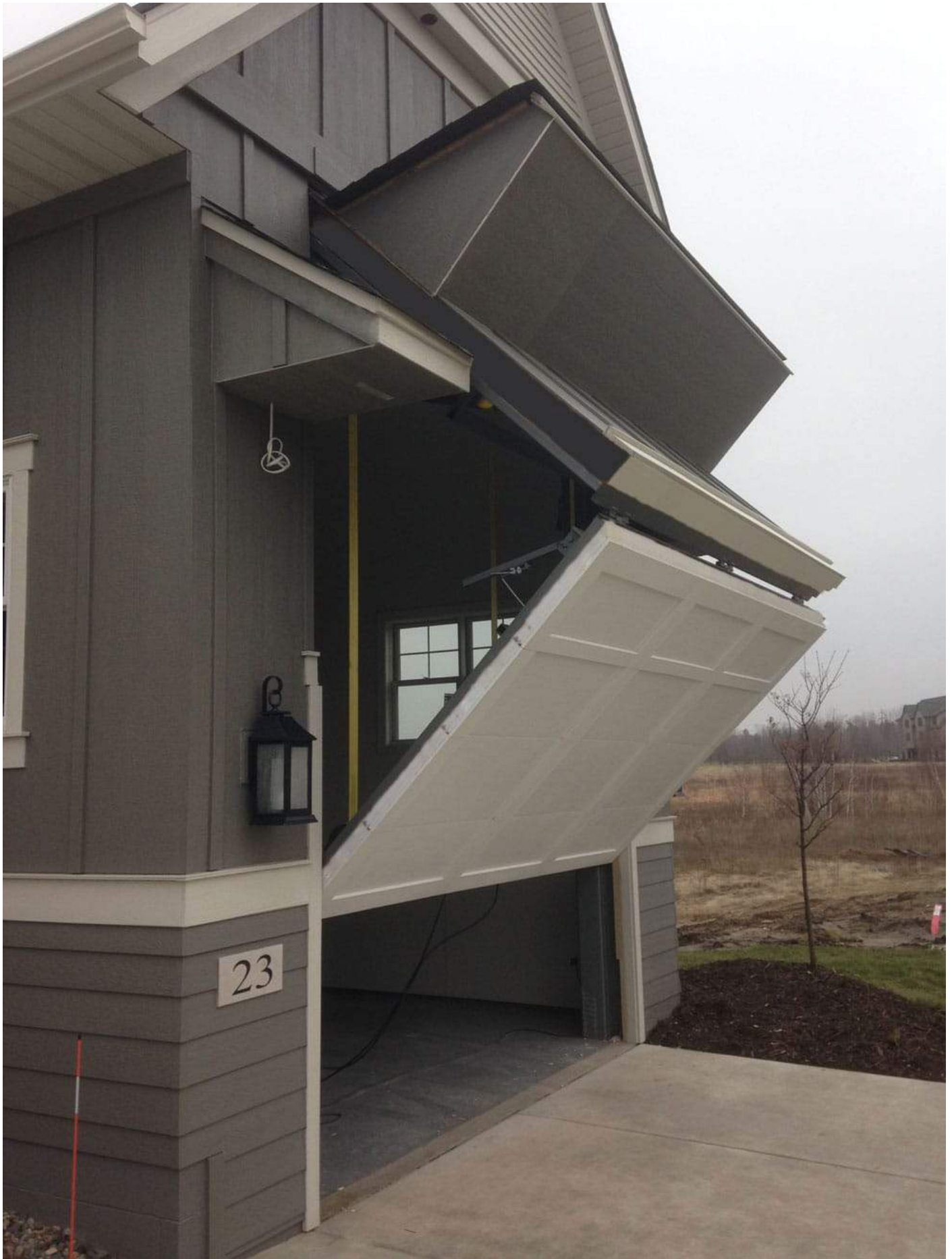
An uninsulated conventional garage door was used to clad the bottom (outdoor) half of the door using LP Smart Siding on the upper half with insulation in the middle of it. Plywood backing sandwiched the insulation on the inside and then it was
