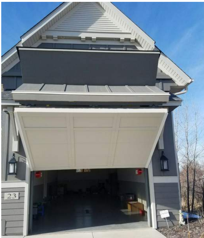
Here you can see how the eave over the Bifold door lifts nicely toward the peak of the garage.
