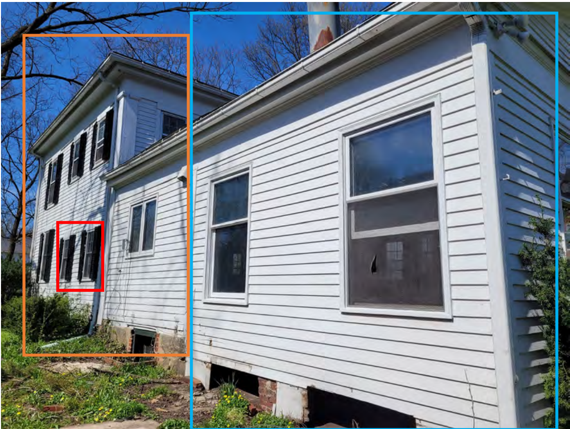
Image 7: Side (west) elevation. The orange block indicates the 1913 addition. The green box indicates the 1925 addition. The blue boxes indicates an addition with an unknown date. The red boxes indicate the vinyl replacement windows.
