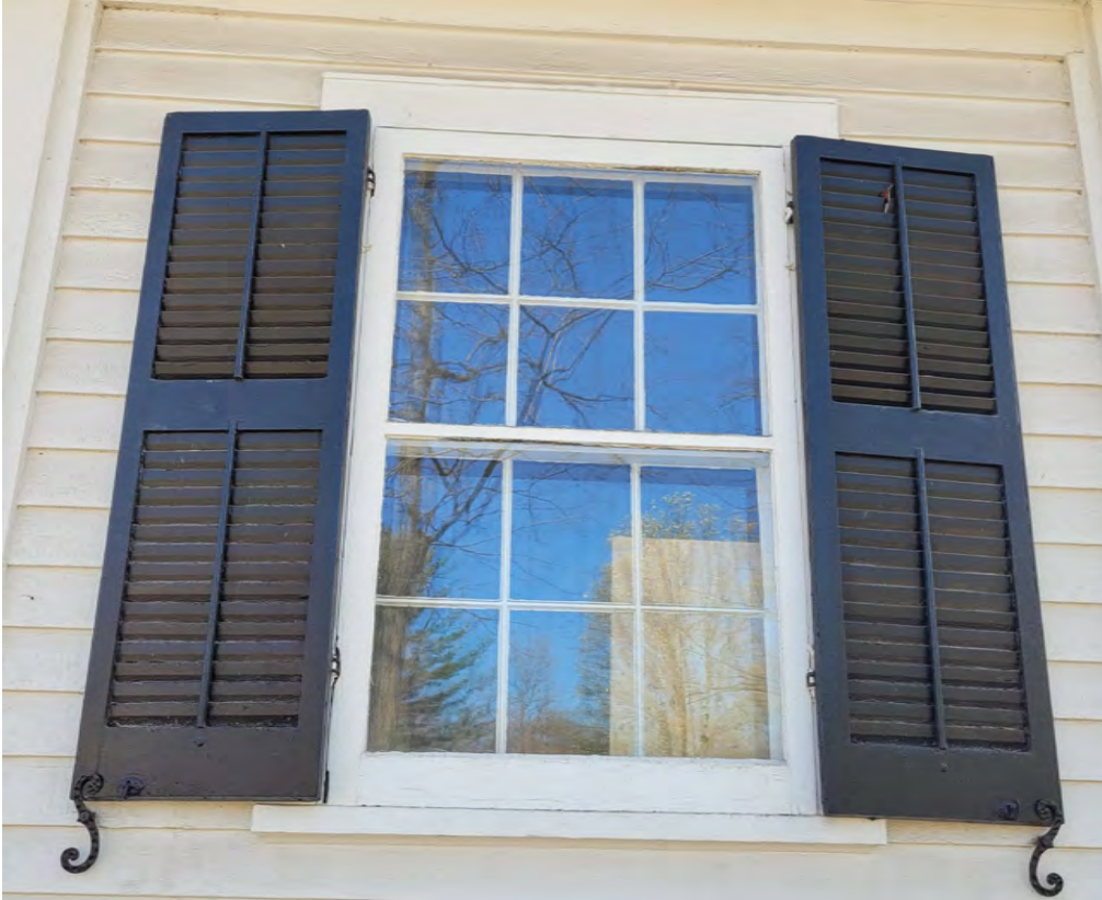
Image 8: Detail of a typical wood window and shutters to be replaced.
