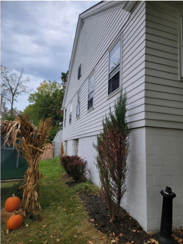
Back of building. No doors.
