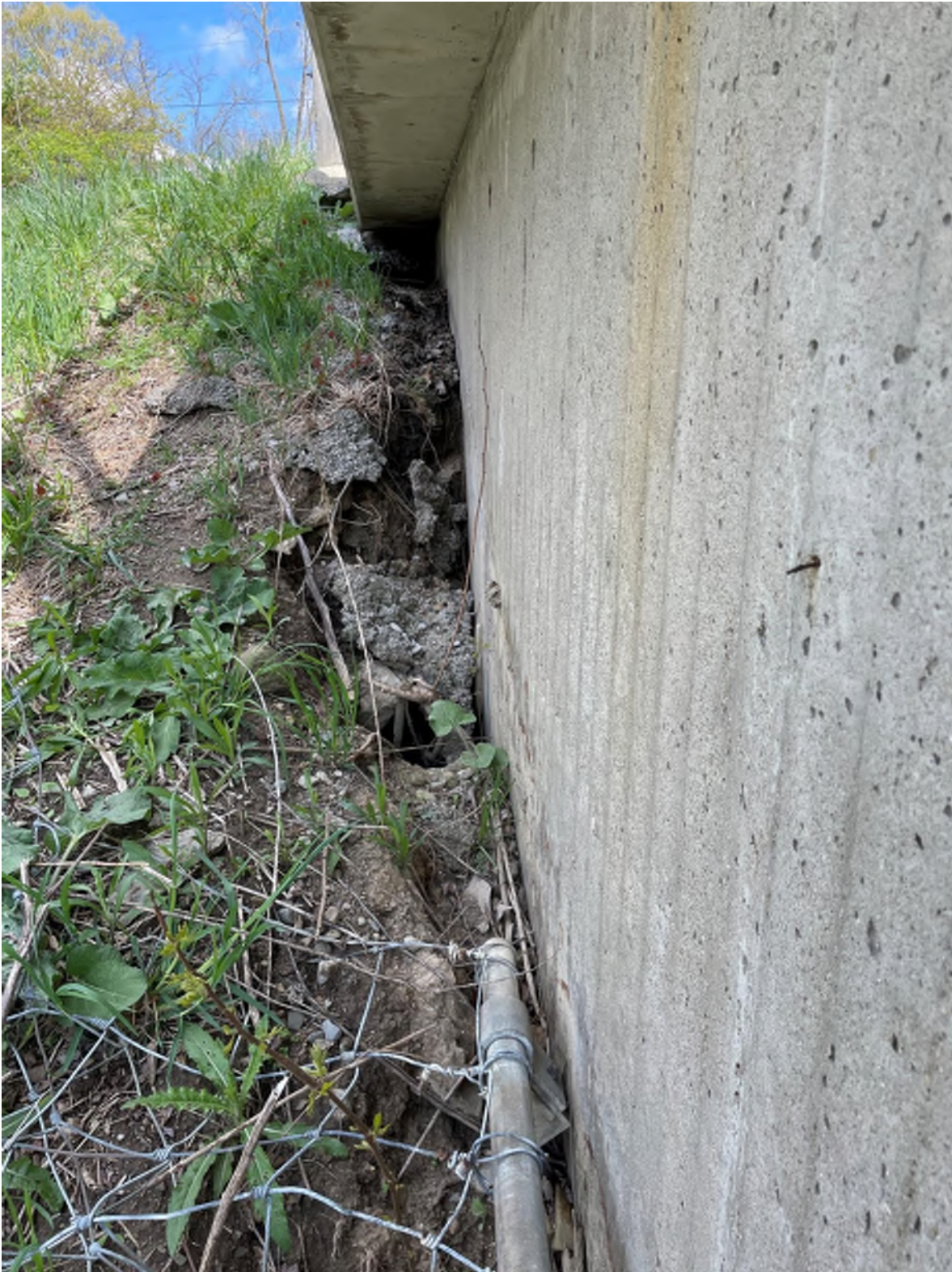
Photograph #10 - Typical Wingwall Condition and Slope Erosion at Forward Left (Northwest) MP 182.1
