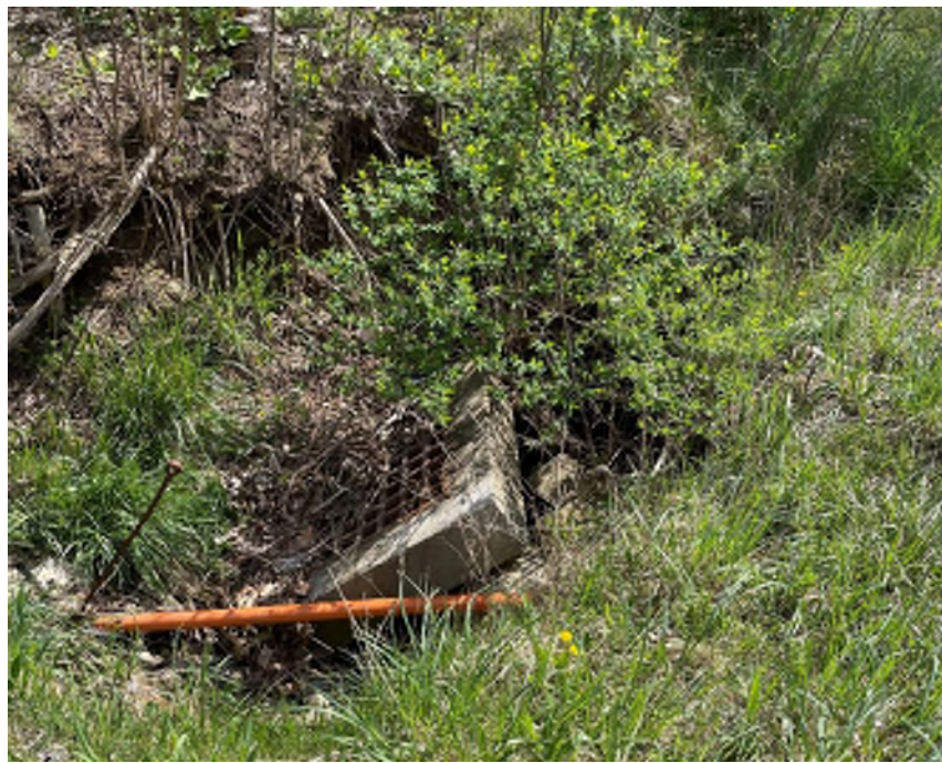
Photograph #9 - Collapsed Forward Right (Northeast) Catch basin MP 182.1
