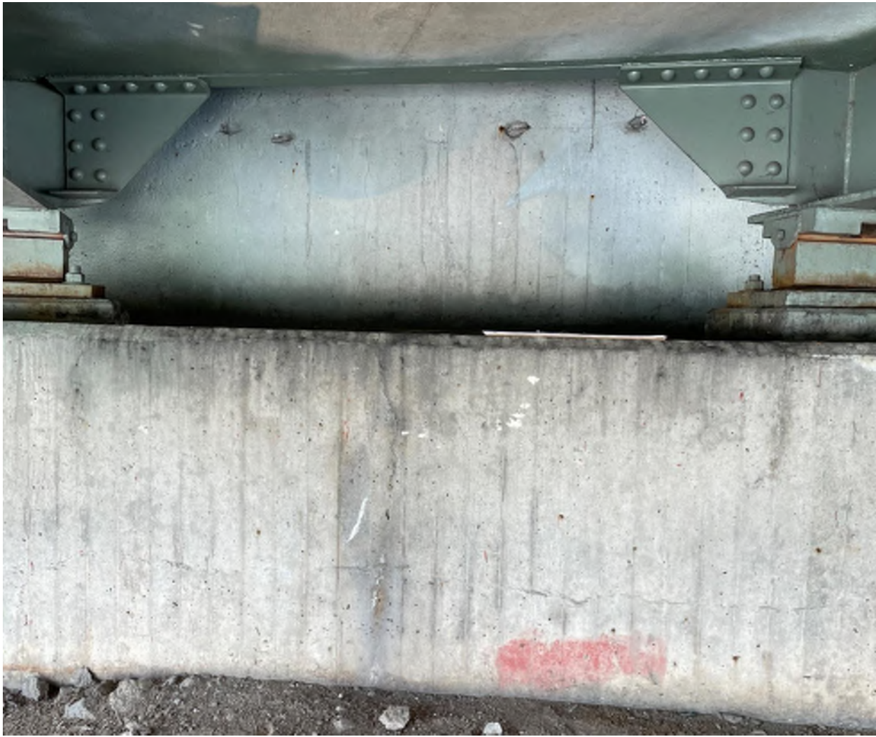
Photograph #7 - Rear (South) Abutment Vertical Crack MP 182.1
