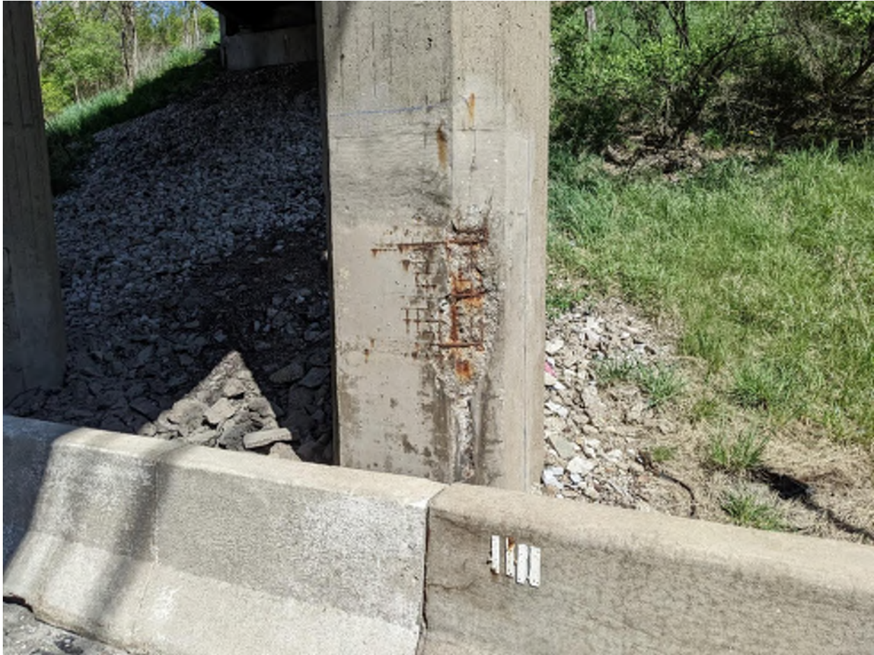
Photograph #12 - Pier 3 Column 3 Spall MP 182.1
