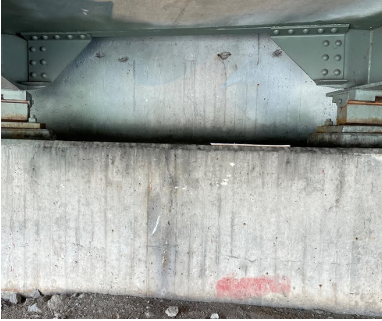
Photograph #8 - Forward (North) Abutment Vertical Crack MP 182.1
