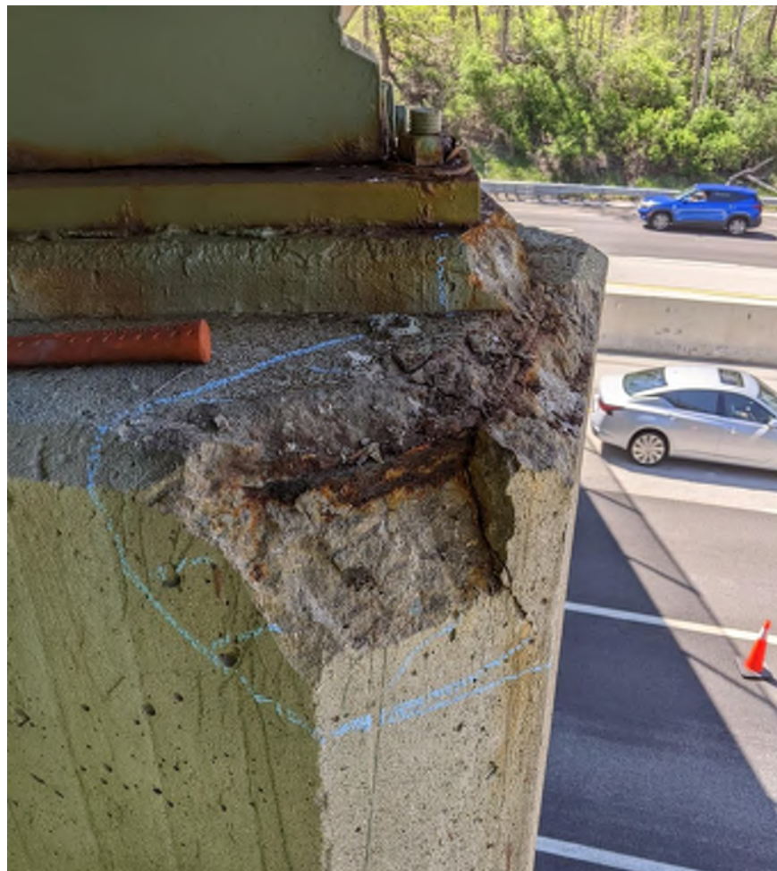
Photograph #12 - Pier 3 Column 3 Spall MP 182.1
