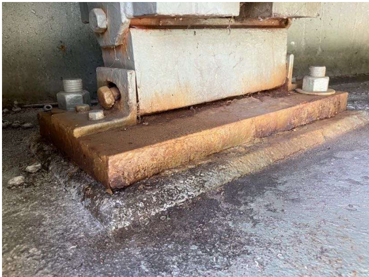
PHOTO 3 View of steel bearing. No gasketing material observed.
