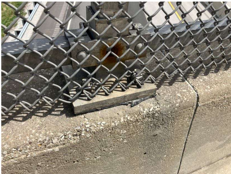
PHOTO 6 View of the vandal fence base plate. Samples taken of caulk material.
