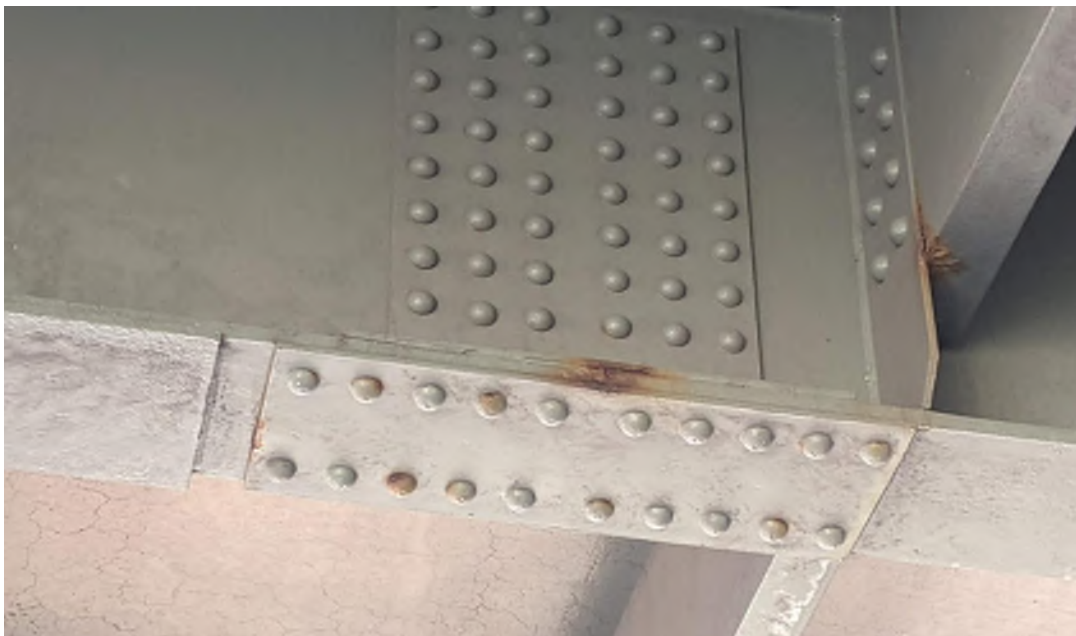
Photograph #5 - Beam 2 Splice with Light Rust, Span 1 MP 182.1
