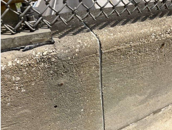
PHOTO 4 View of typical joint on parapet wall. Samples taken of caulk material.
