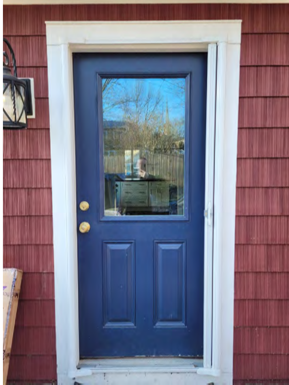
Image 7: Detail of rear (north) door to be reinstalled on the rear (north) elevation in the new side (east) one story mass.
