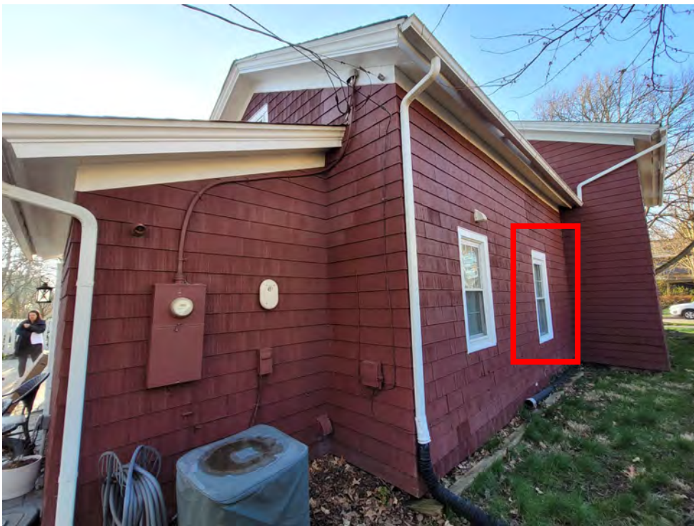
Image 6: Side (west) elevation. The red square indicates the non-historic vinyl window that is proposed to be reused.
