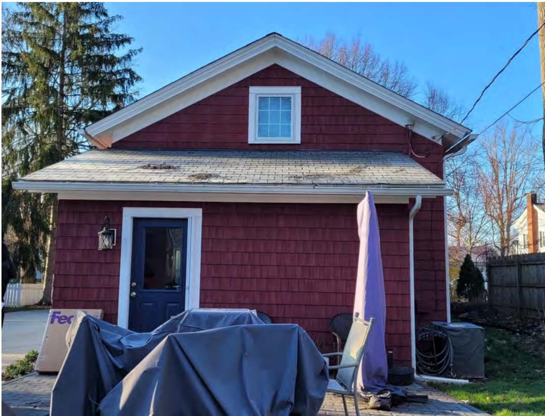
Image 4: Rear (north) elevation. The one-story mass will remain in place, but the roof will be removed and replaced. The second-floor window will remain.
