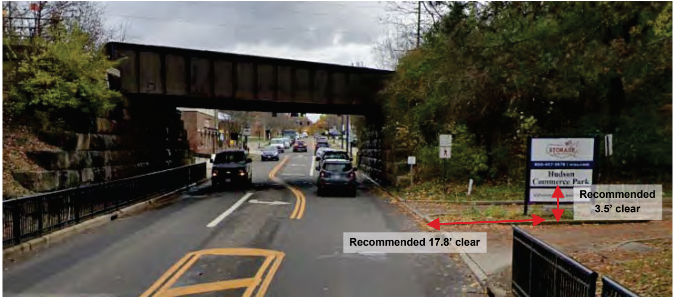
Figure 4: Sign blocking sight distance
