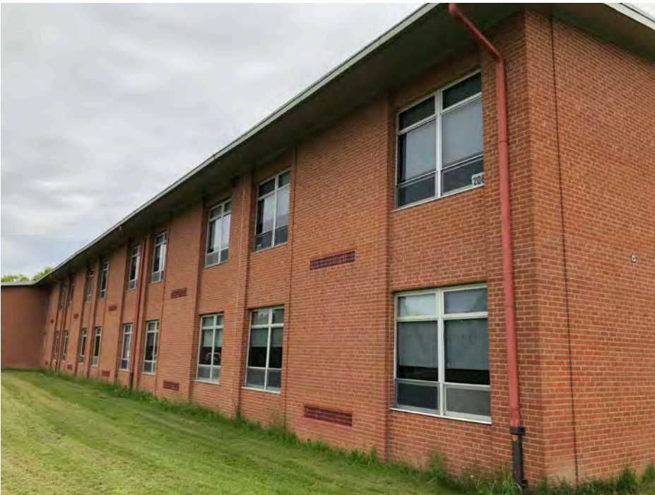
East side of the 2-story wing – the 2-story classroom wing to be connected at this location
