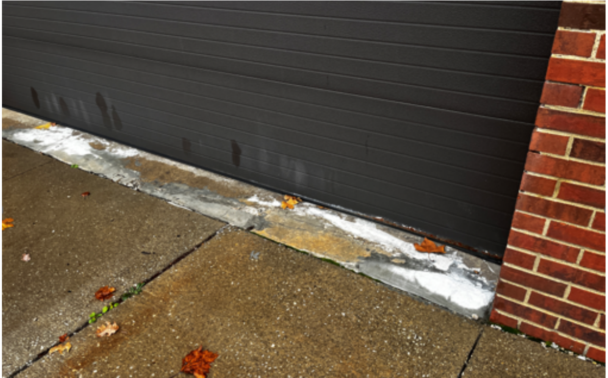
REPAIRS FROM SALT AT APPARATUS BAY OVERHEAD DOOR
