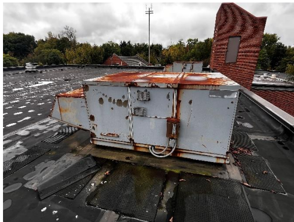
APPARATUS BAY HEATING VENTILATING UNIT
