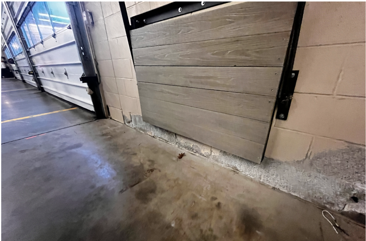
APPARATUS BAY CMU DETERIORATION FROM SALT
