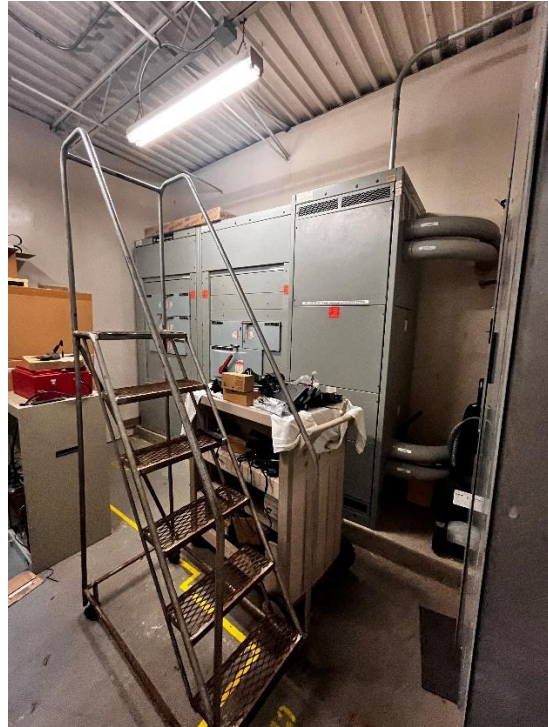
MAIN DISTRIBUTION PANEL
