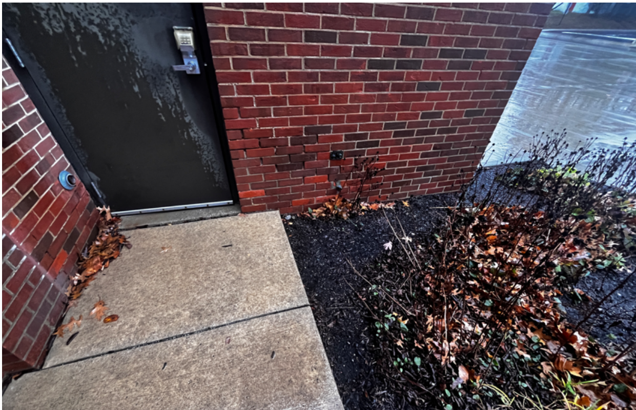
EXTERIOR WALL REPAIRS & CONTINUOUS DAMAGE DUE TO LACK OF WATERPROOFING
