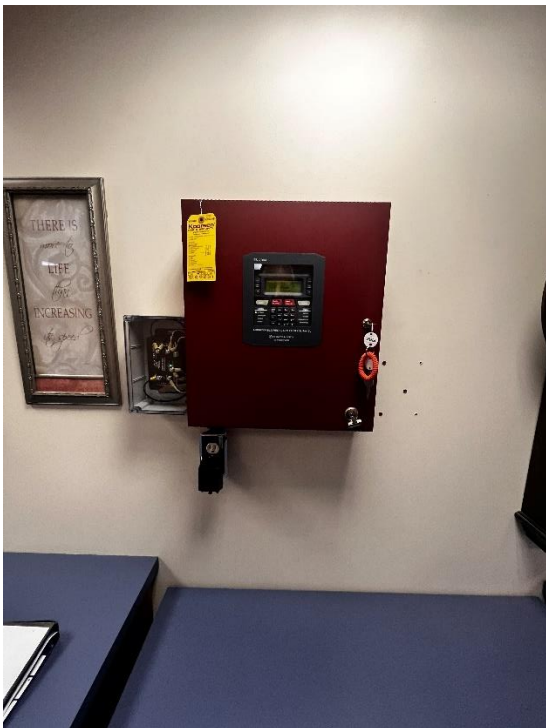
FIRE ALARM CONTROL PANEL
