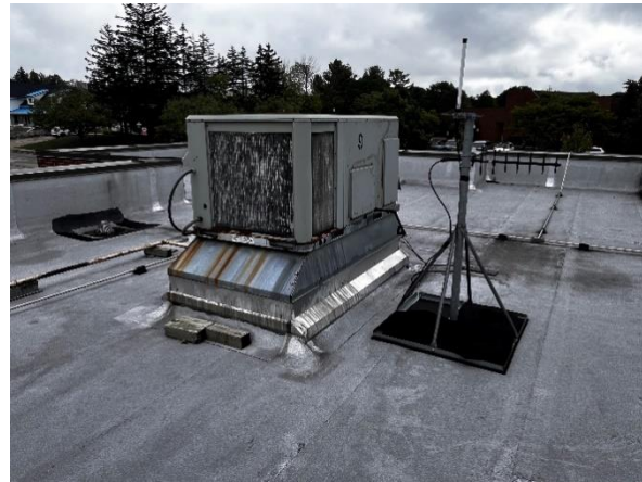
TRANE DX ROOFTOP UNIT #9
