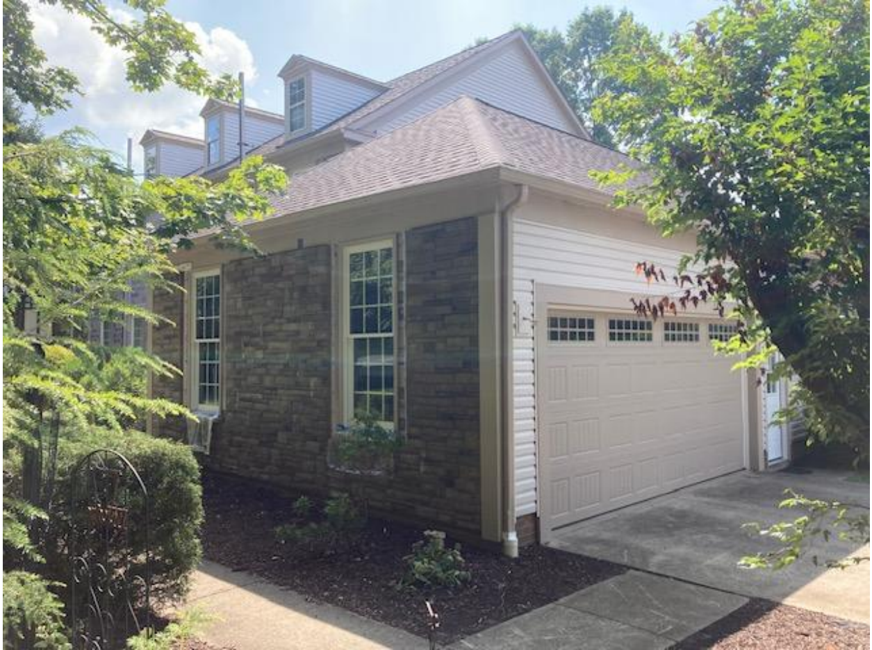
North side transition to West side: Corner posts upgraded from wood to wood-grained AZEK of same color.
