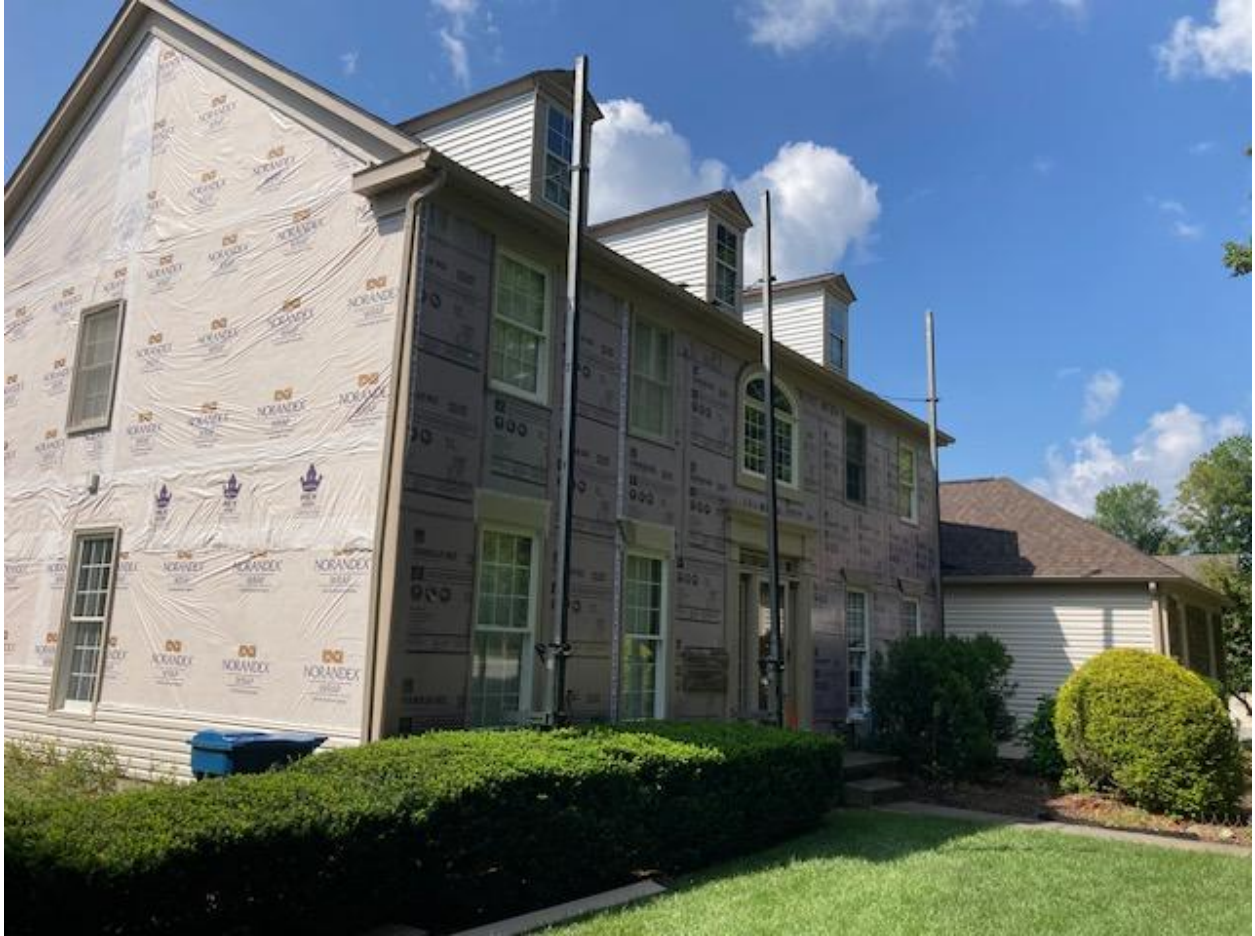
East side transition to North side: Vertical trim board upgraded from wood to wood-grained AZEK of the same color.
