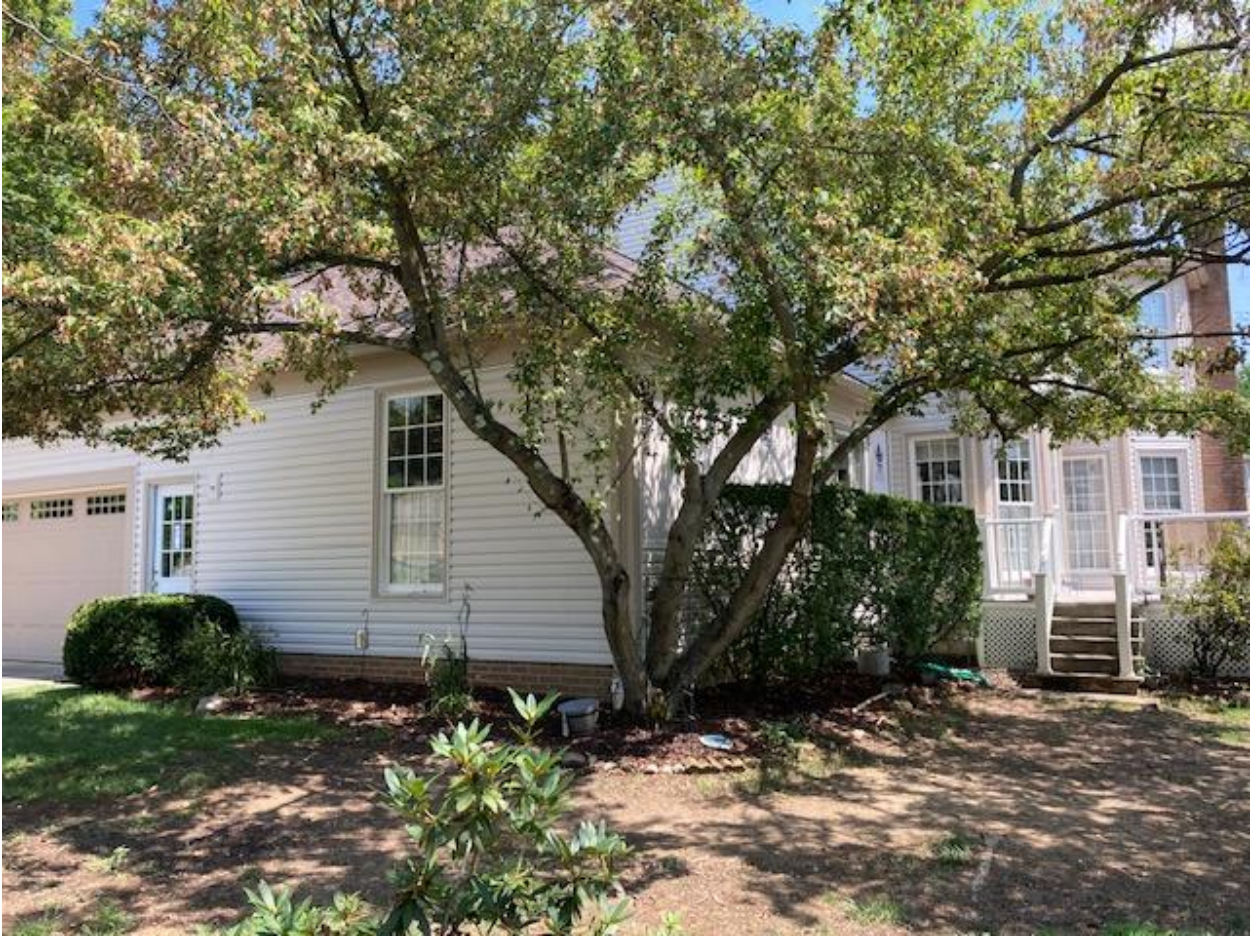
West side transition to South side: Corner post upgraded from wood to wood-grained AZEK of same color.
