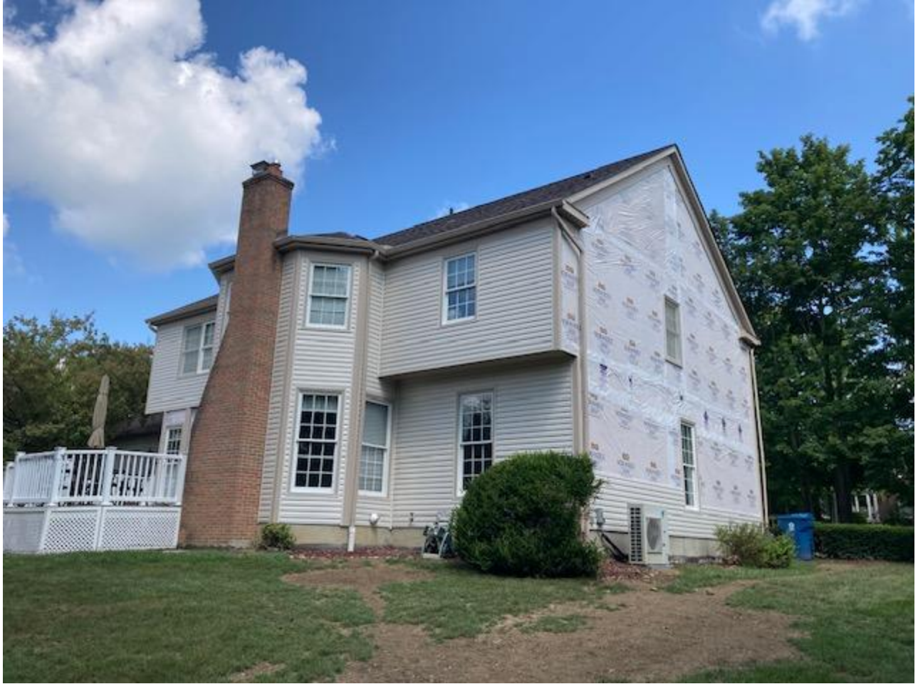
South side transition to East side: Corner posts upgraded from wood to wood-grained AZEK of the same color.
