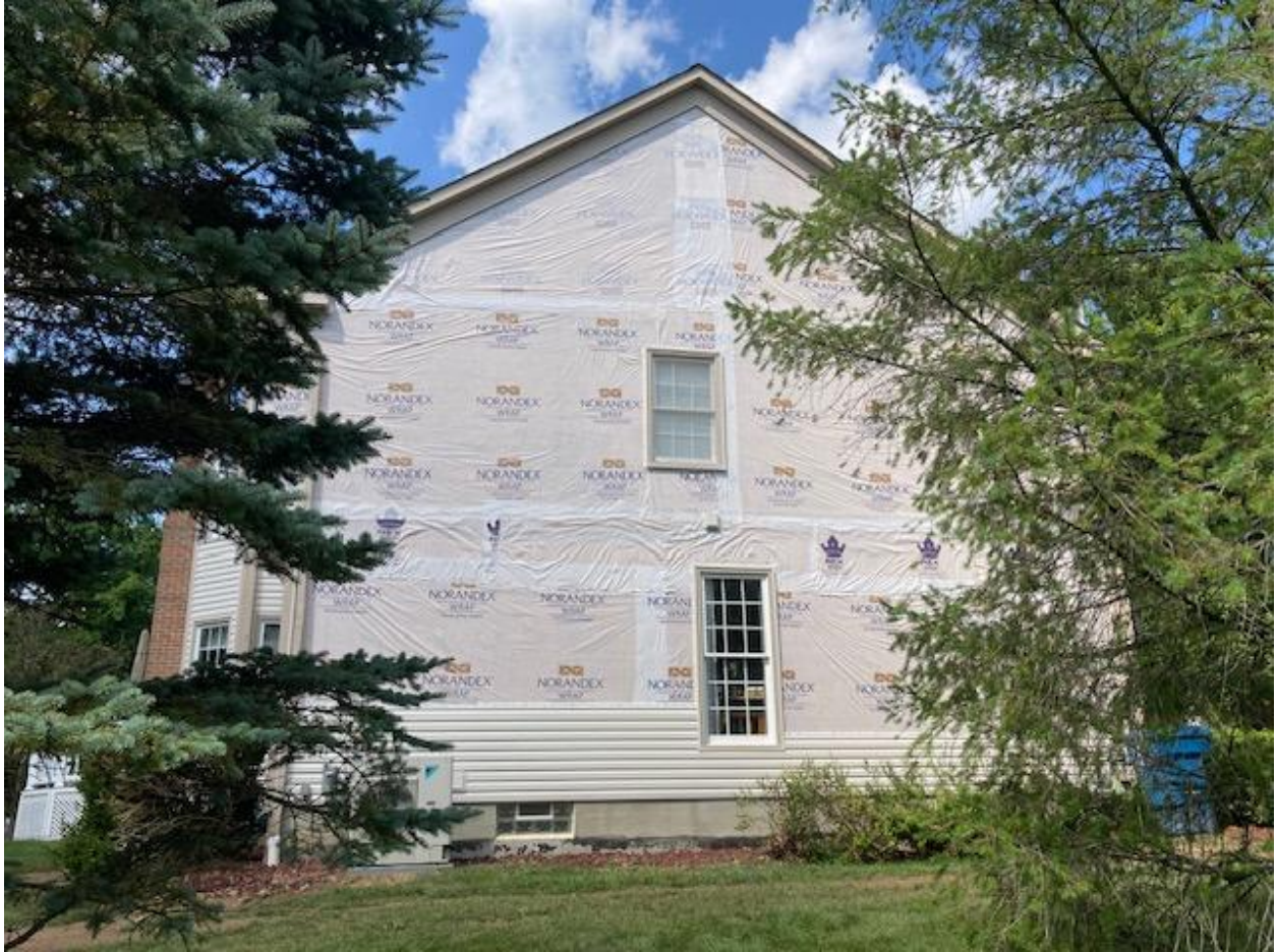
East side: Aluminum siding replaced with insulated vinyl siding of same style and color. Frieze boards upgraded from wood to wood-grained AZEK of same color.
